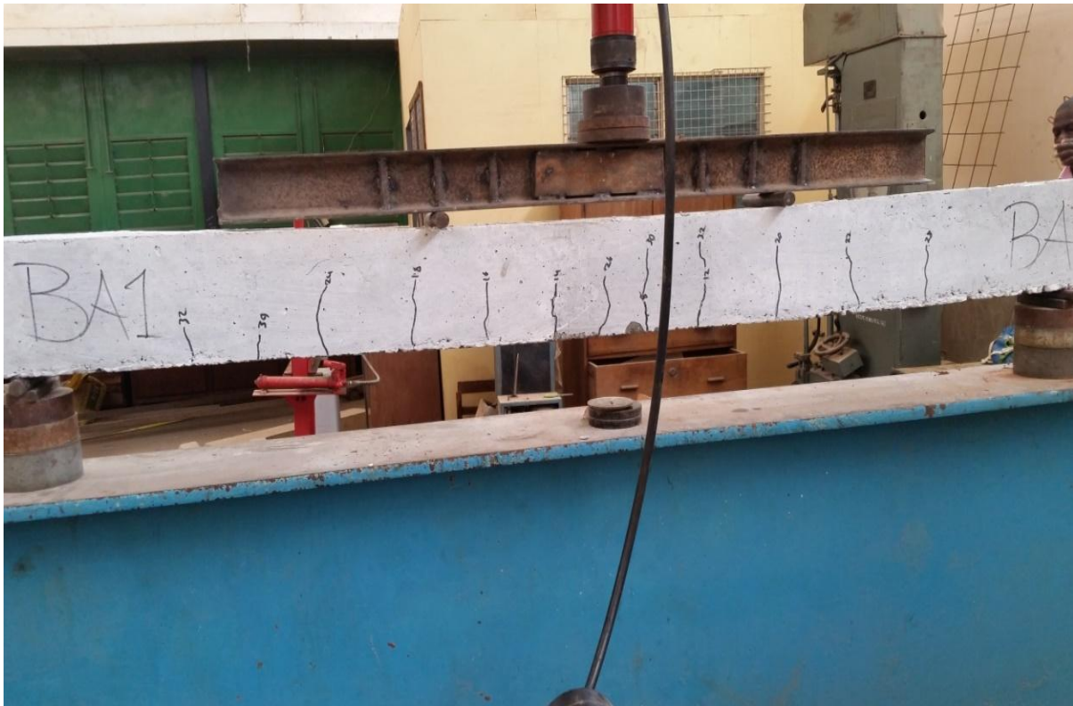
Fig. 4. Crack propagation of the control specimen
